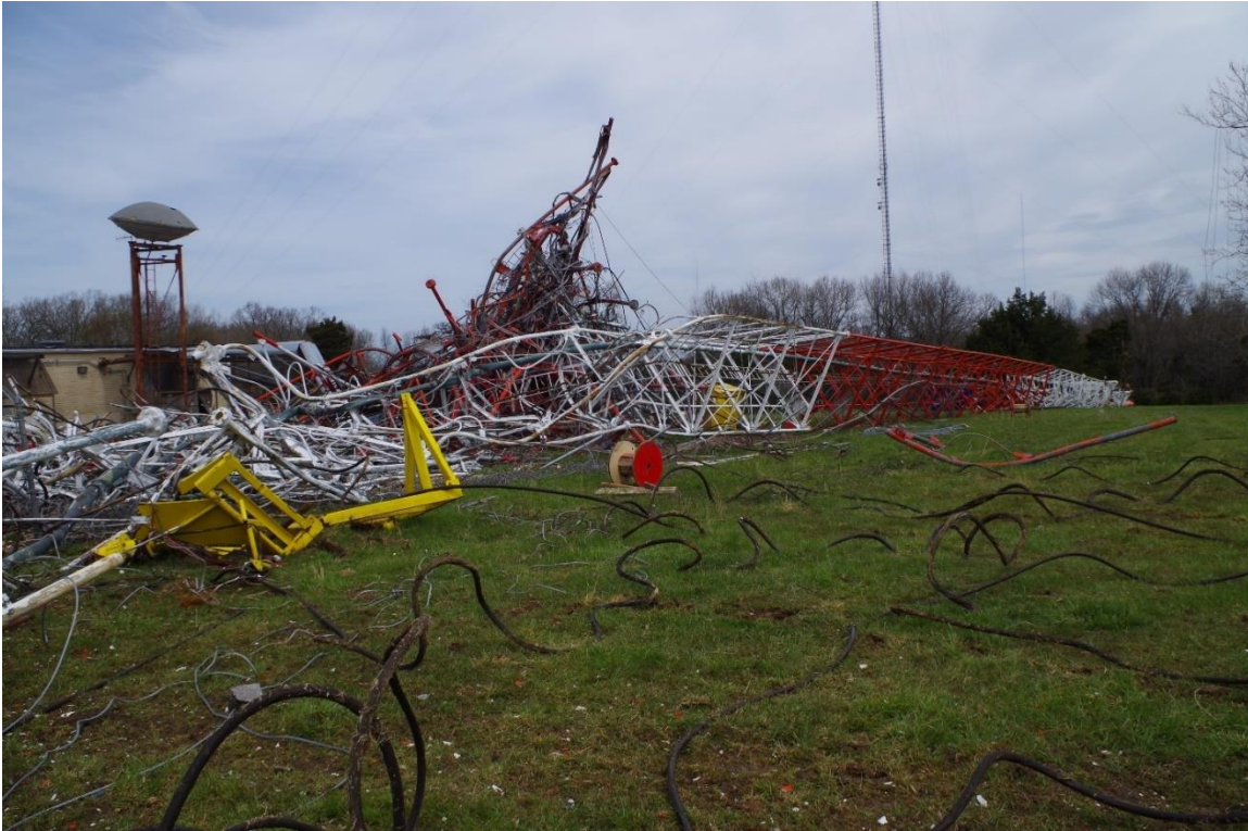
Figure 6 Top Section of Collapsed Communication Tower
