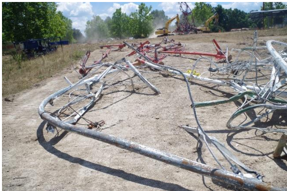
Figure 8. Bent Tower Leg from the Recovered Section
